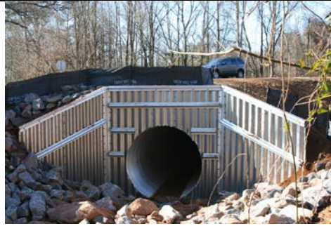
Use Pipe Wingwall
