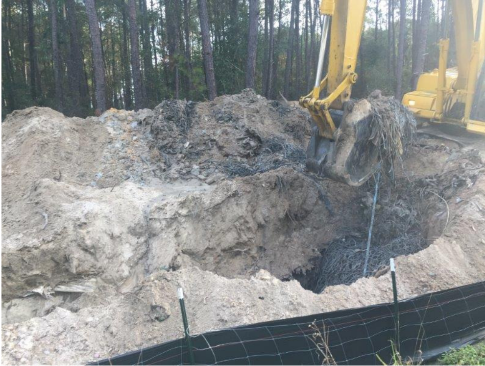
Photograph 3: Typical view of fan belts located within most of the test pits.
